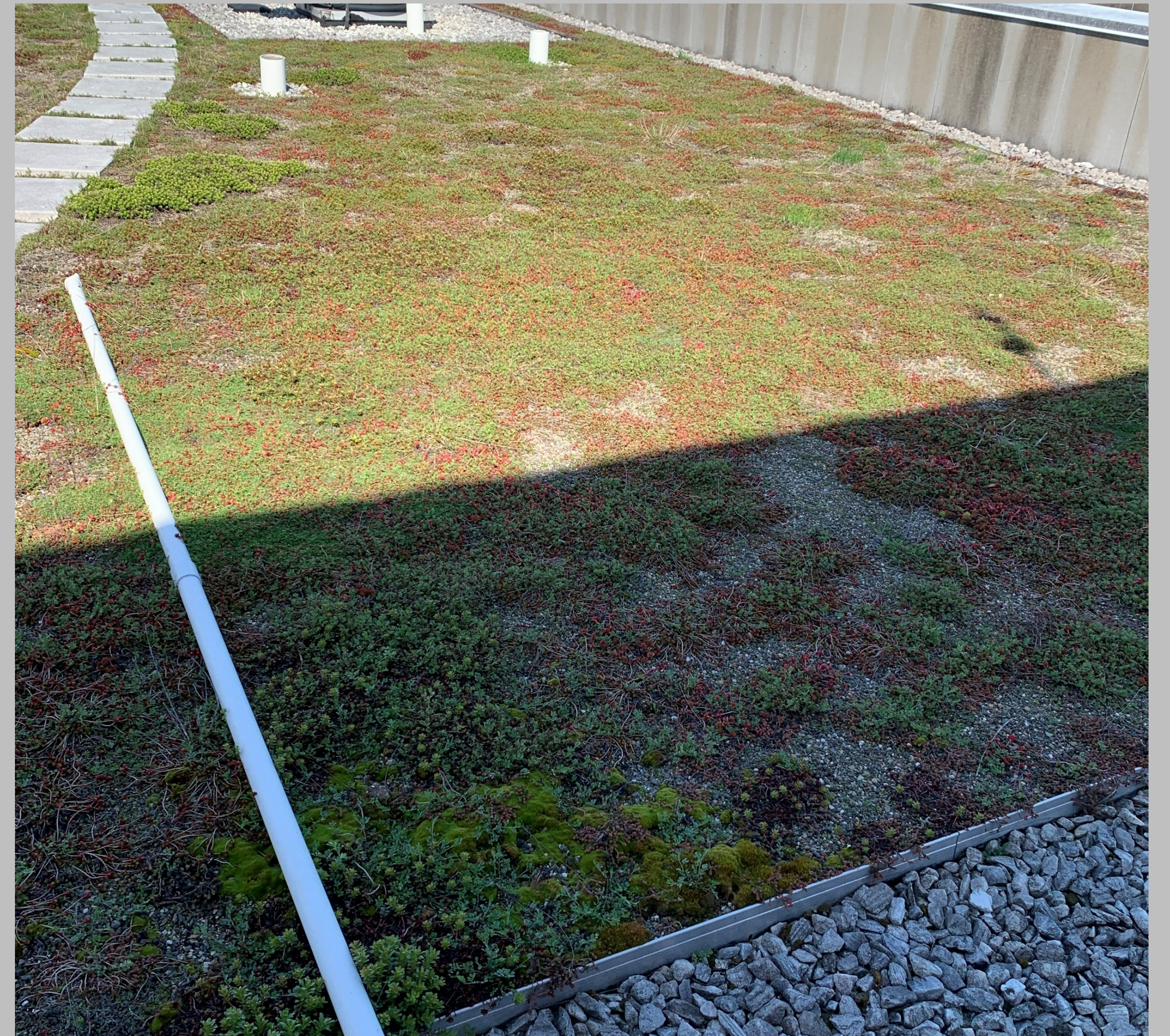
This is the green roof on the top of Cumberland that collects rainwater from storms.
